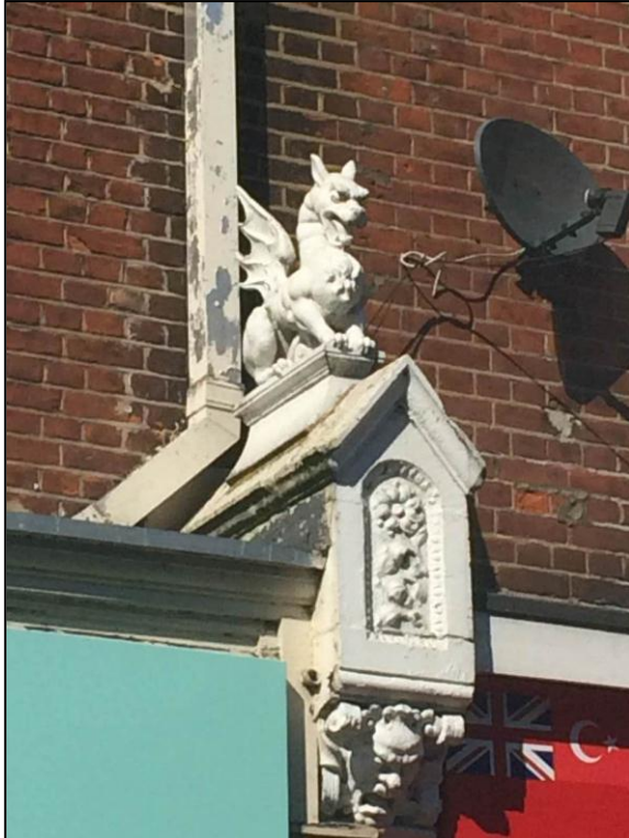
Griffon detail with satellite dish and peeling paint
