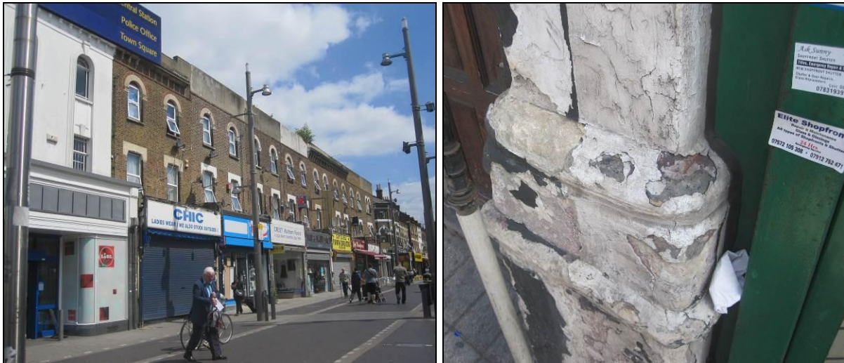
Figure 45: Vegetation growing on parapet and deteriorated plaster
