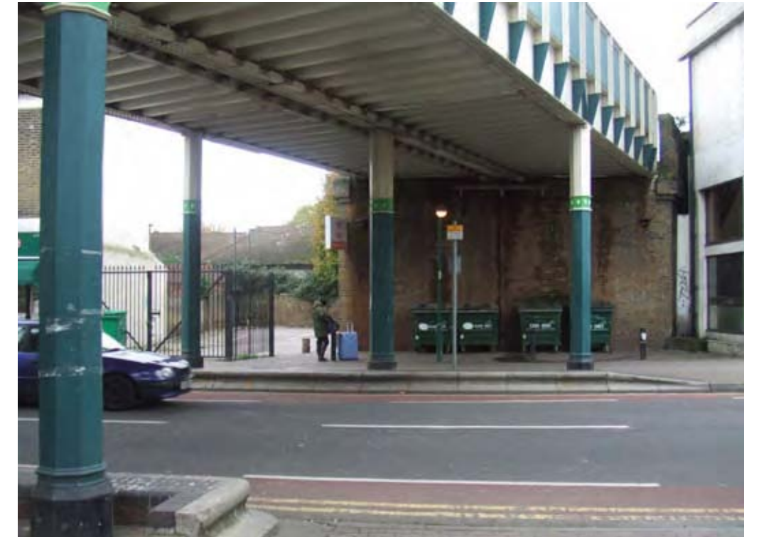
Poor quality access point
