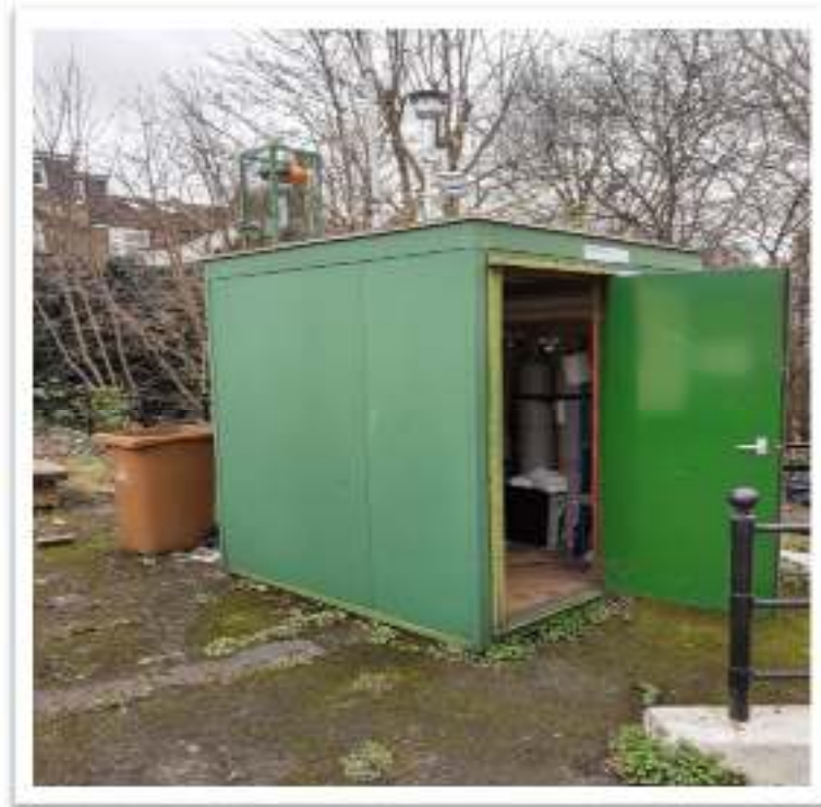
Real time Air Quality Monitoring Equipment, Dawlish Road E10
