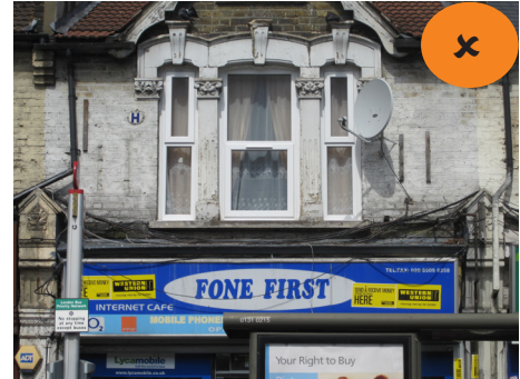
Poorly sited wiring and other clutter can detract from the quality of the facade
