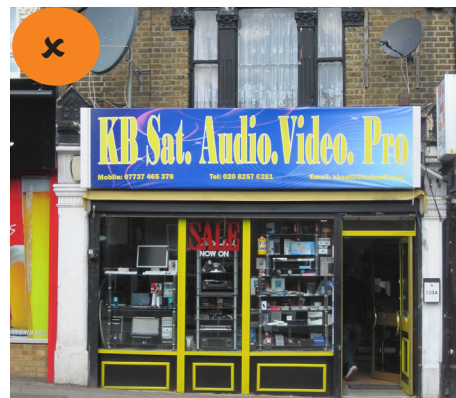
This fascia sign is overly large and extends above the sill of the first floor window
