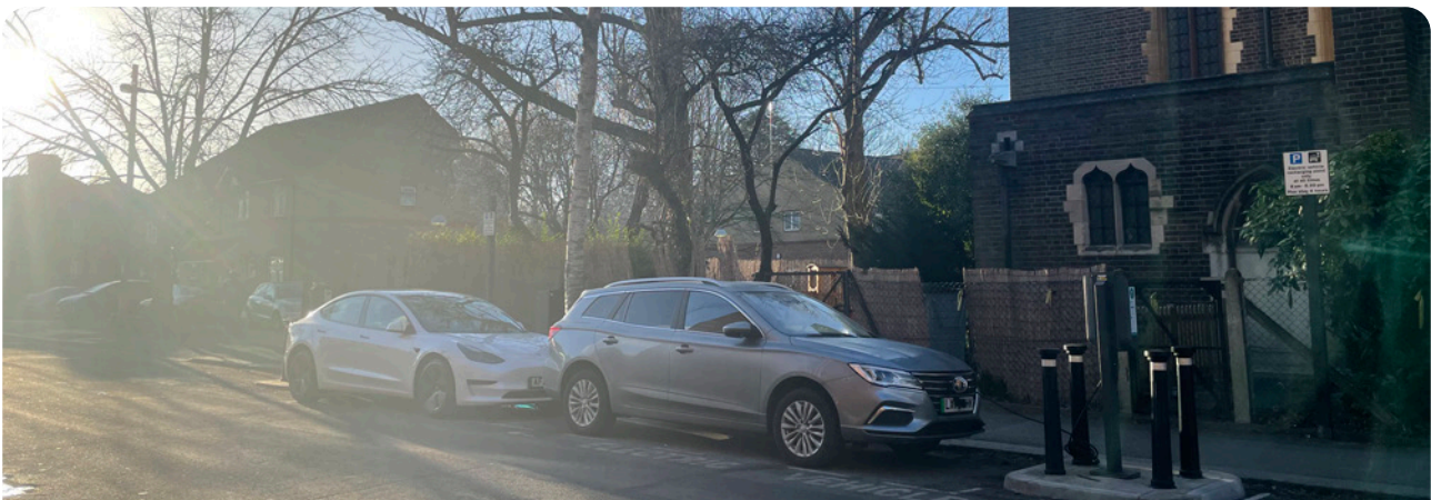
FAST 22KW DUAL SOCKET CHARGING POINT ON BROOKSCROFT ROAD, E17
